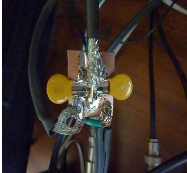
Shack end of coax showing capacitors and ground wires to going the radios and computer.
